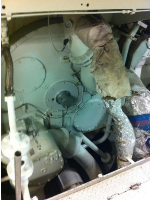
CPS mounted on engine / in engine room
